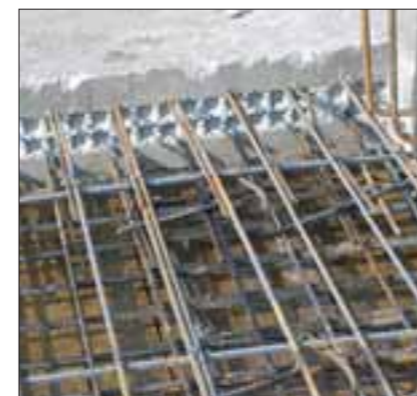
In small manholes in the bridge deck, it's an improvement to have denticulations, made in a simple and neat way.
